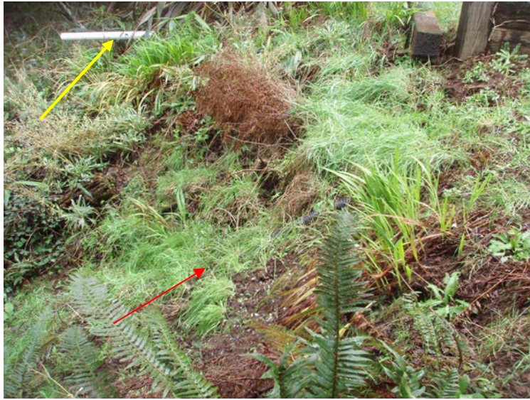
Drainpipes (center and upper left) discharging to slope. Vertical post in upper right is on east boundary of subject property.
