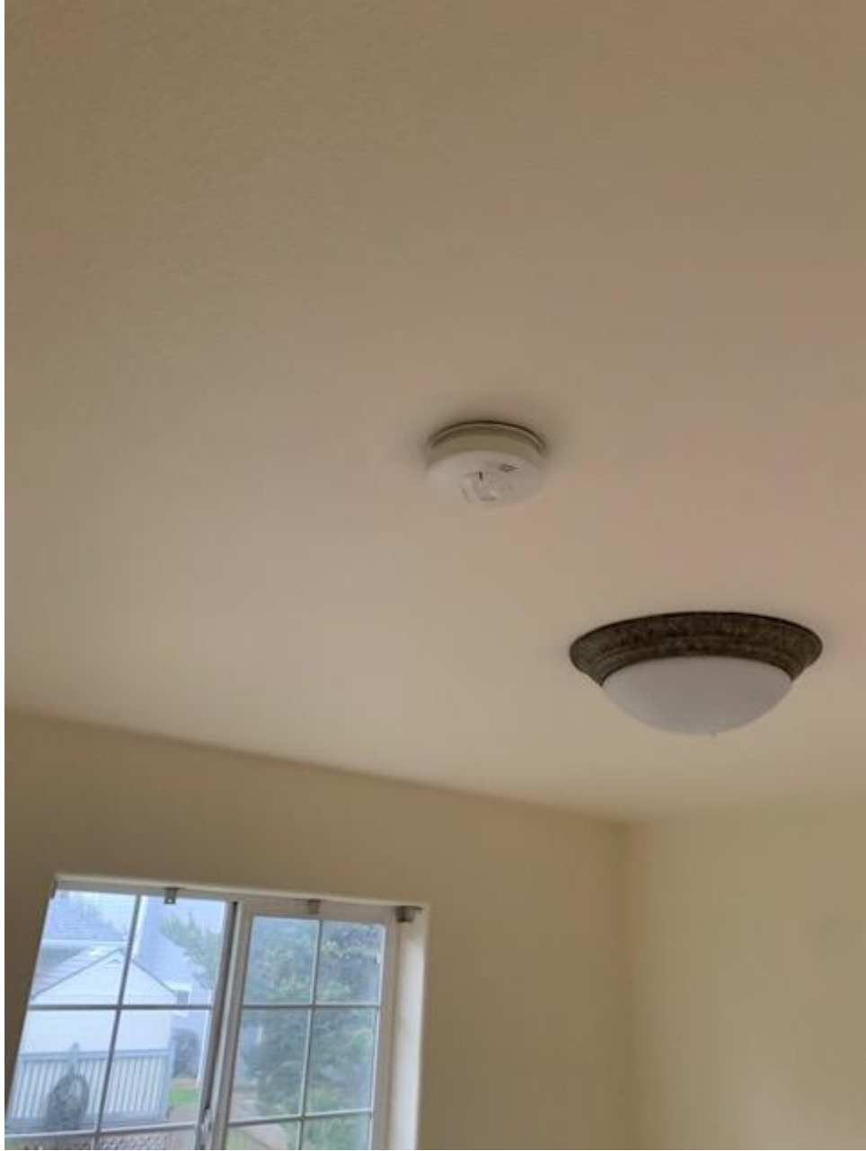
Smoke alarm in bedroom #2
